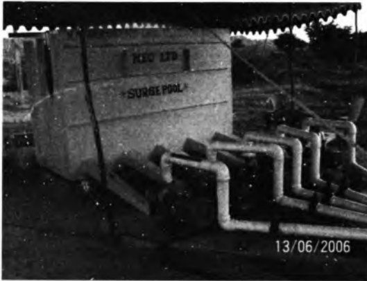
Photo 7 Draft tubes, pumps & Delivery mains
